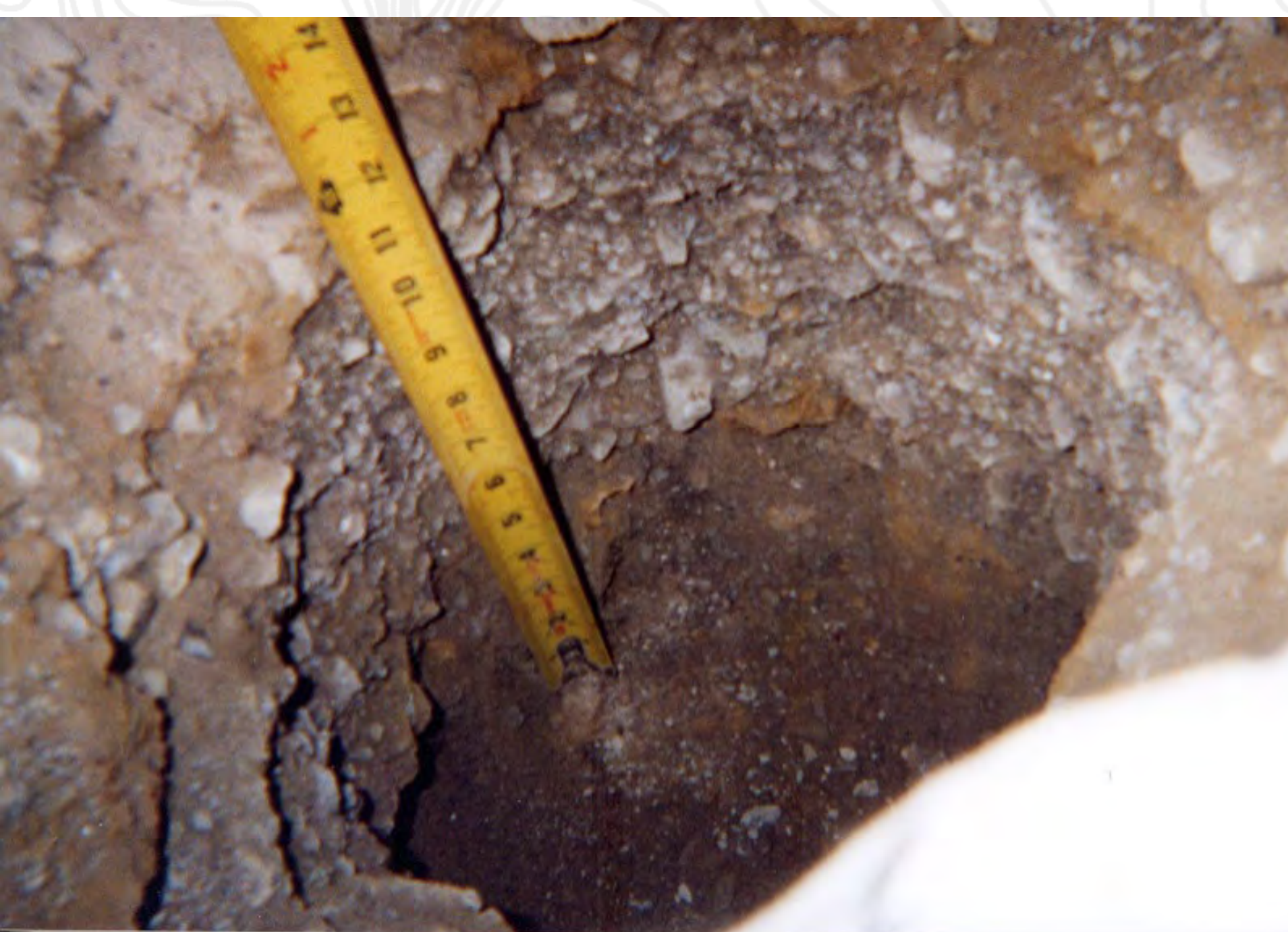
Very Densely Compacted Trench Backfill
