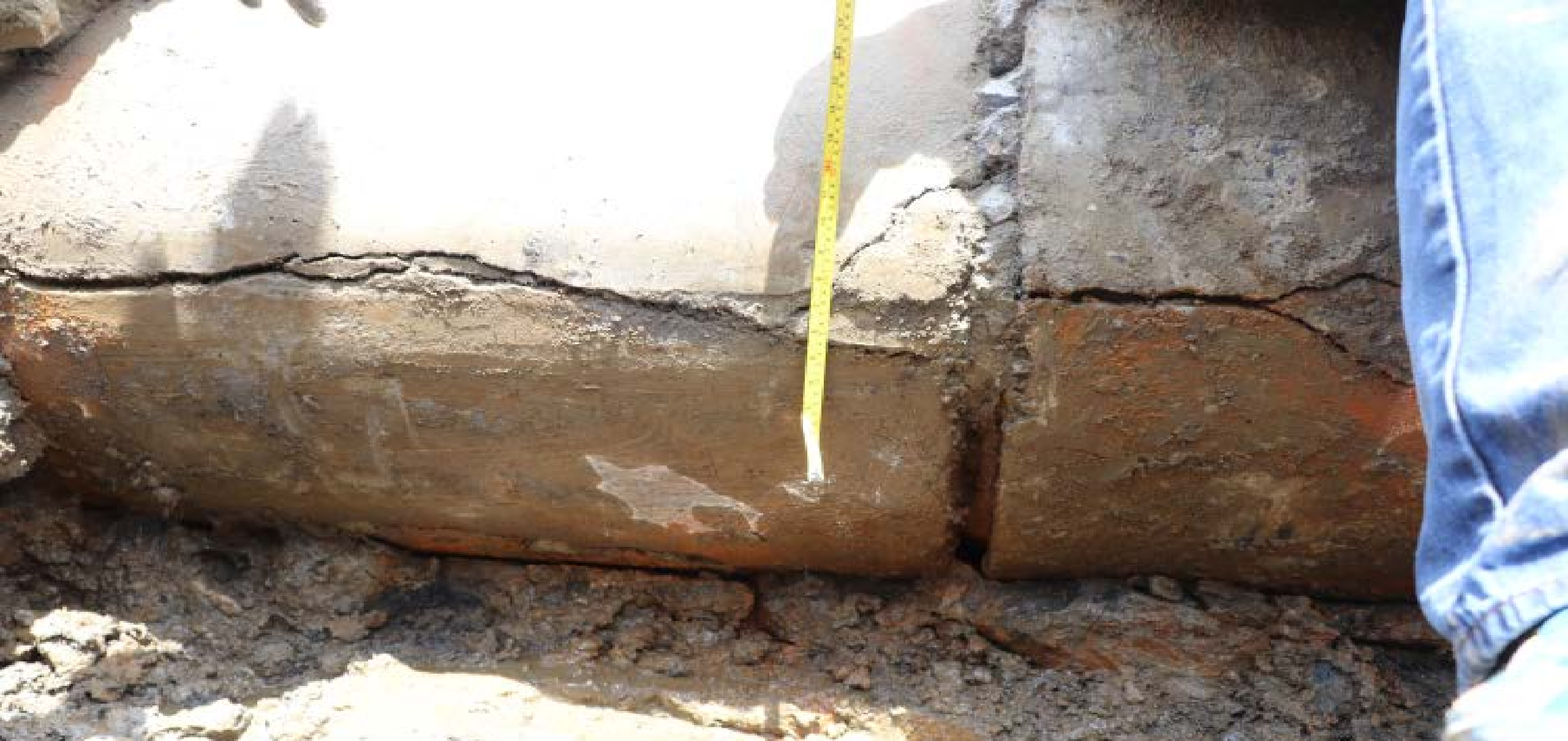
Reinforced concrete conduit affected by non-uniform settlements
