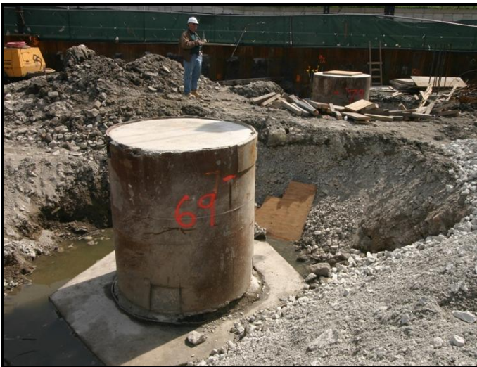
Fig. 19. Top of Caisson 69 (and Caisson 79 in the background) prepared with a high-strength, cased concrete cap for dynamic load testing.
