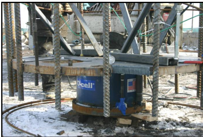
Fig.8. Cage and base plate configuration for a limited base area Osterberg load test on a production caisson.
