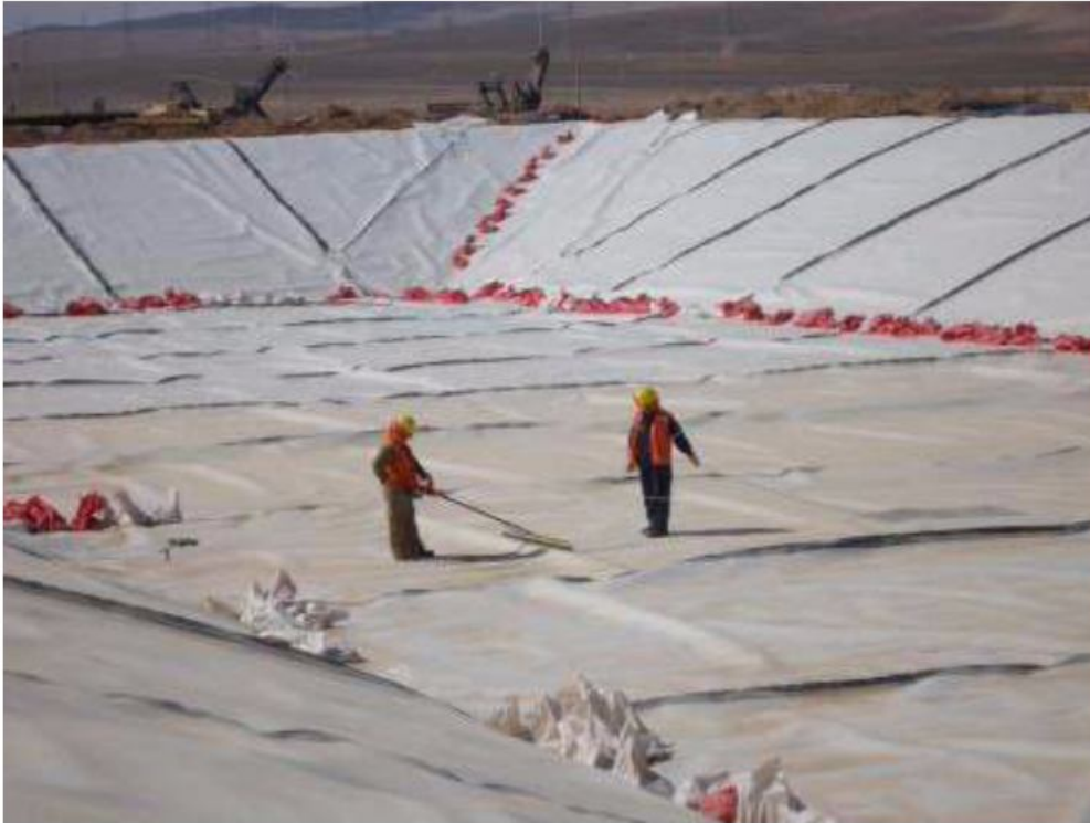
CQA - Leak Location
