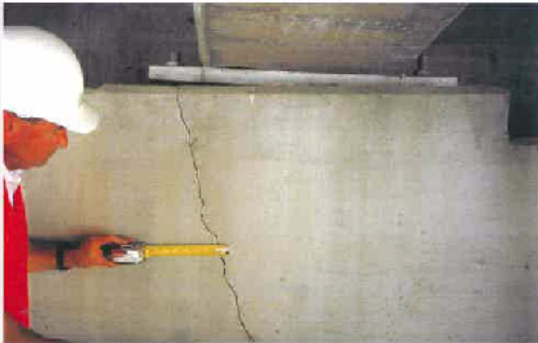
Diagonal Stress Crack in Under Beam
