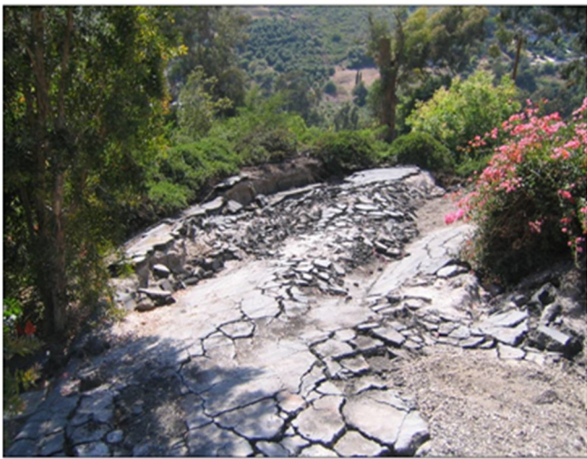
Figure 33 – Severe damage from development of obsequent scarps, caused by toppling towards the left.
