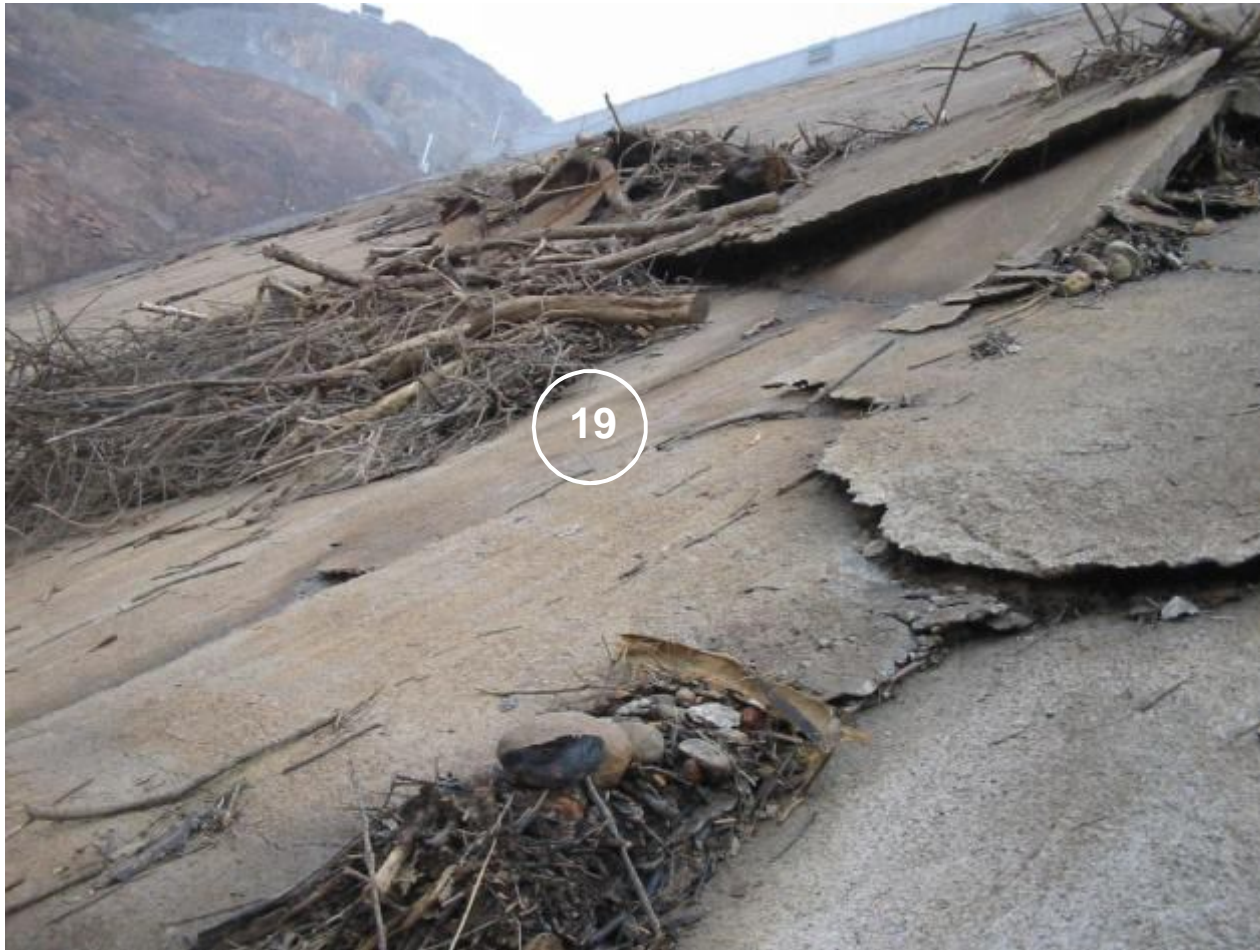
Inclined cracks in slabs 19, 20, 21, 22
