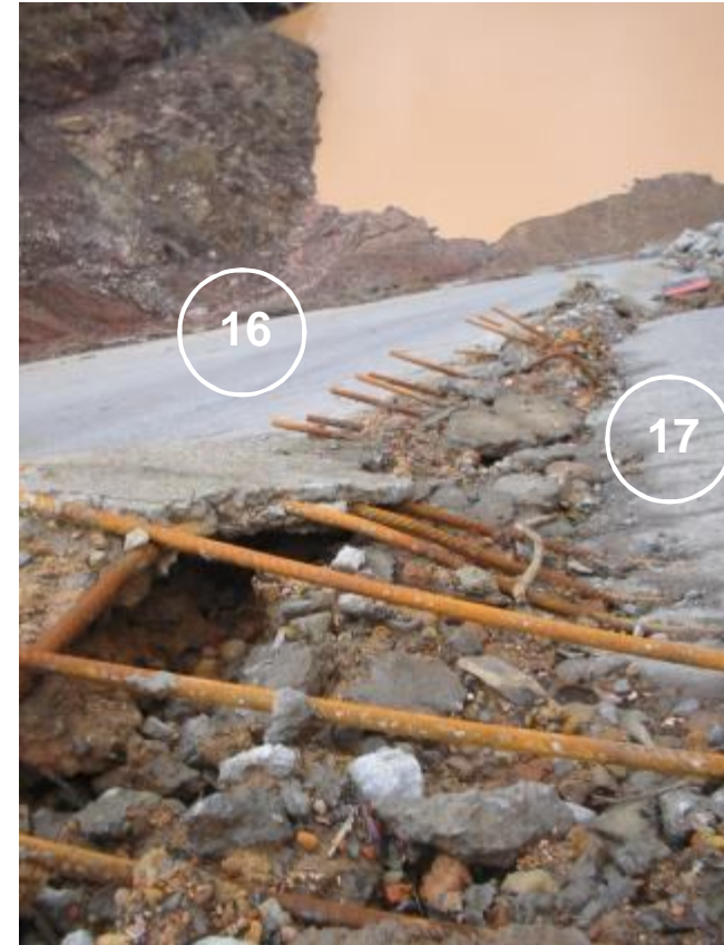
ZONE CLOSE TO THE INCLINED CRACK IN SLAB 17
