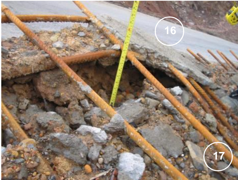
CONCRETE RAISED UP -26 CM
