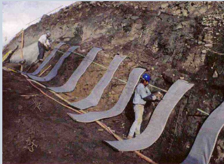
Use of continuous and intermittent geocomposite back drains when using fine grained soils in the reinforced soil zone (compl., TenCate Geosynthetics, Inc.)
