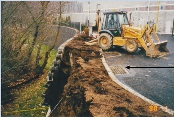
Surface water drainage inlet
