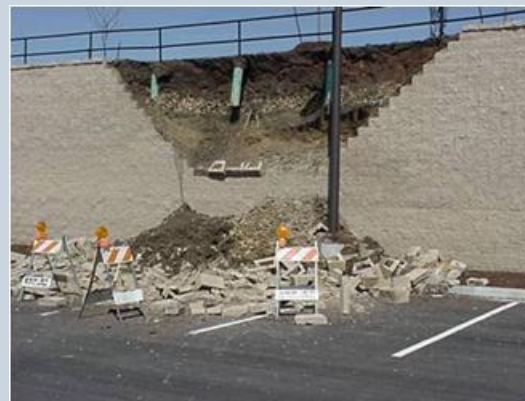
Tension Crack Behind
