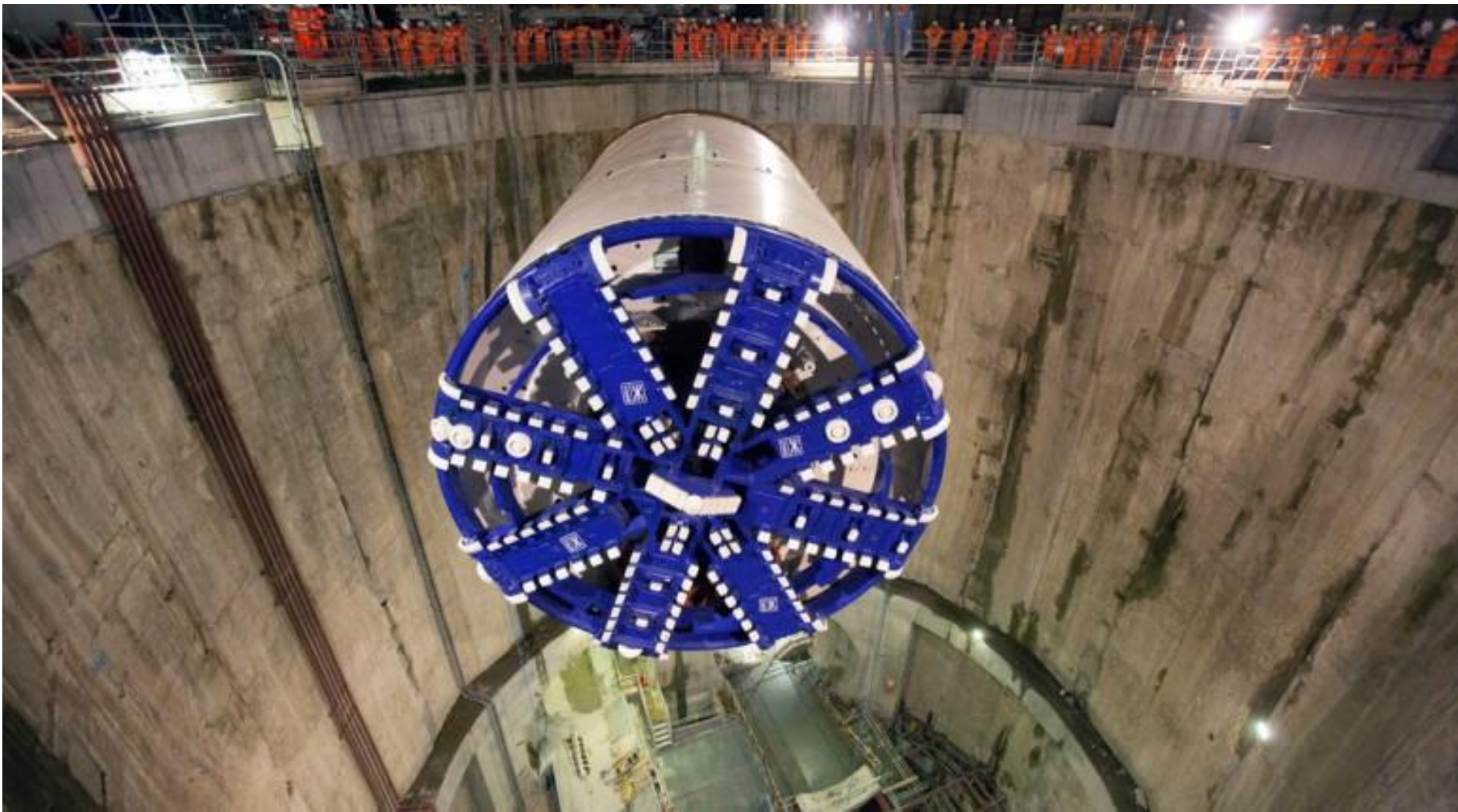
Crossrail – 550 tonne tunnelling machine Elizabeth being lowered into 40m deep shaft at Limmo Peninsula
