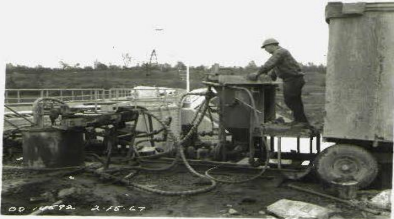
Photo No. 31. Grouting equipment. High speed, double drum grout mixer is on right; agitator is on left. Grout pump is behind agitator. View towards left abutment.
