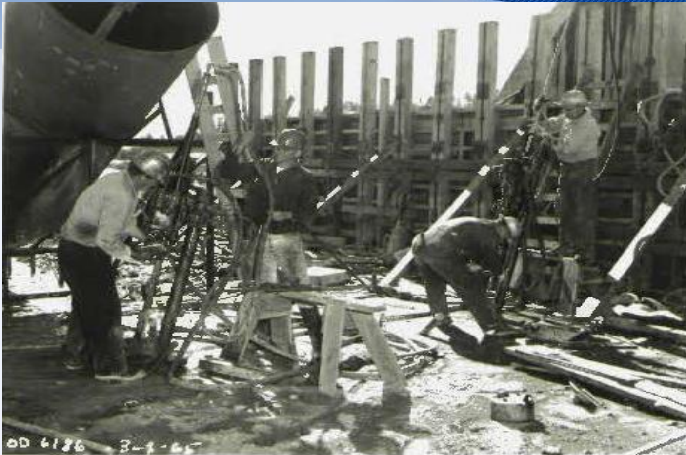
Photo No. 30. Drilling curtain holes through concrete at Elevation 188 in monolith 19. View downstream. Neg. No. OD 6186 2-4-65
