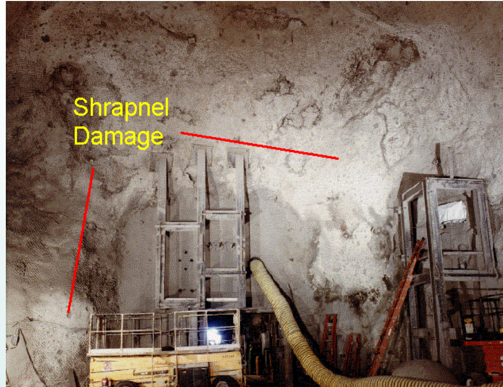
Observed damage – Shotcrete spalling
