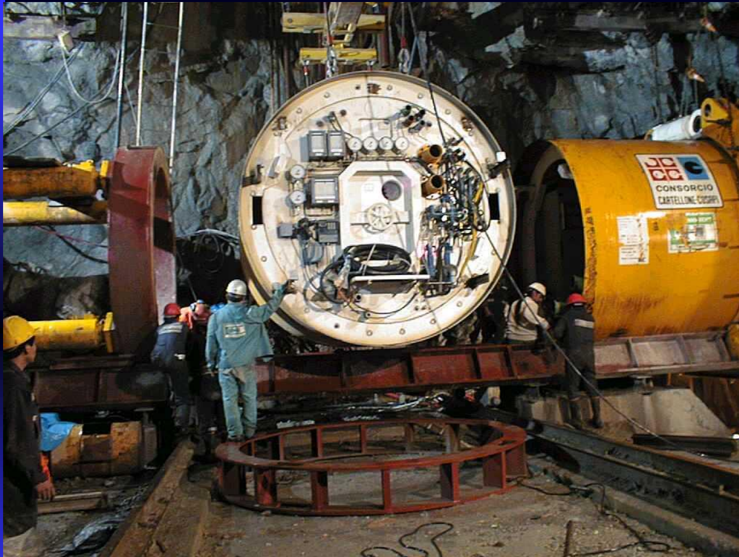
ASSEMBLY OF THE MACHINE IN THE LAUNCHING CAVERN ON THE RIGHT BANK
